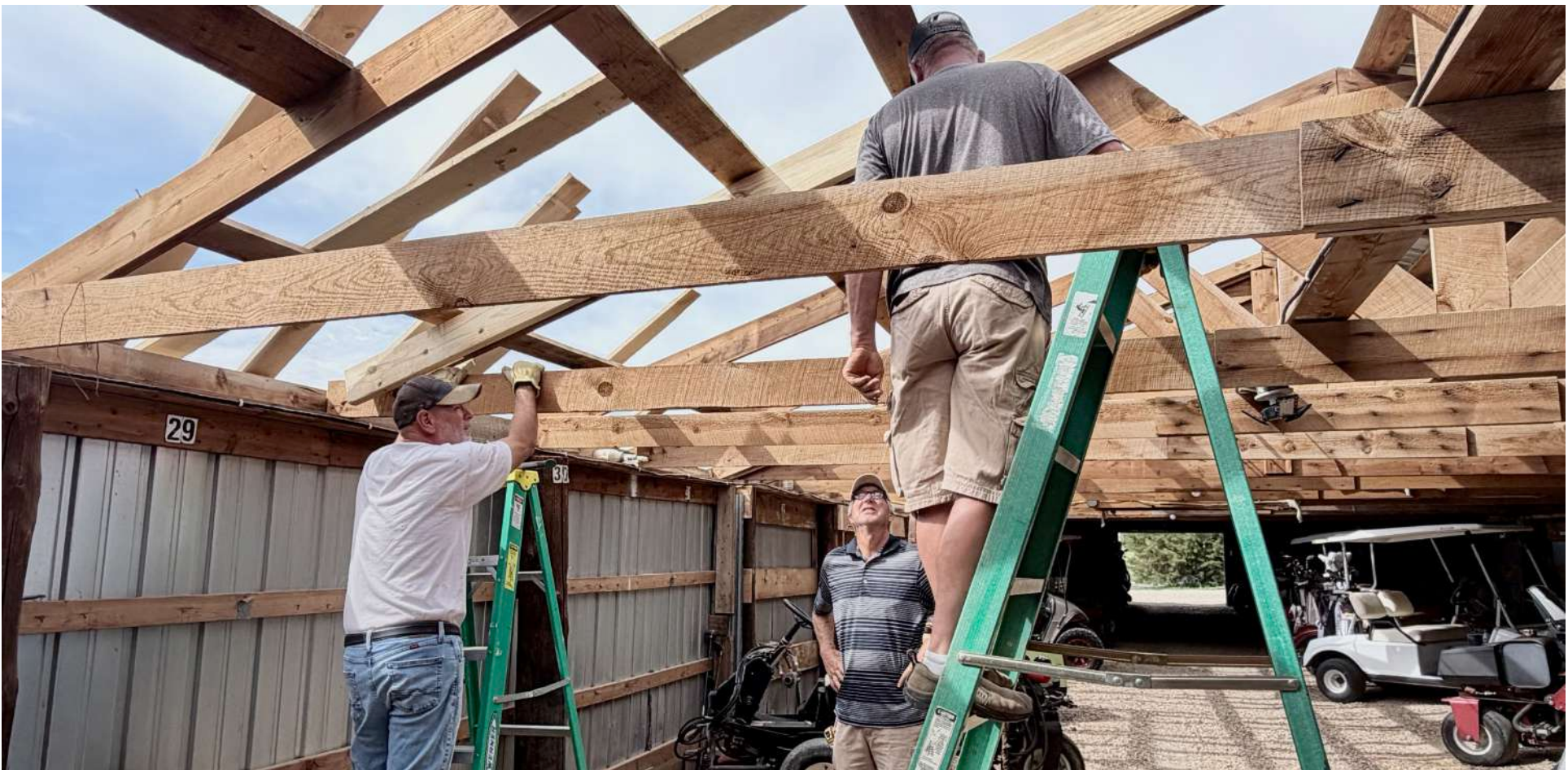
Making a plan to fix the roof. Longbrake photos
