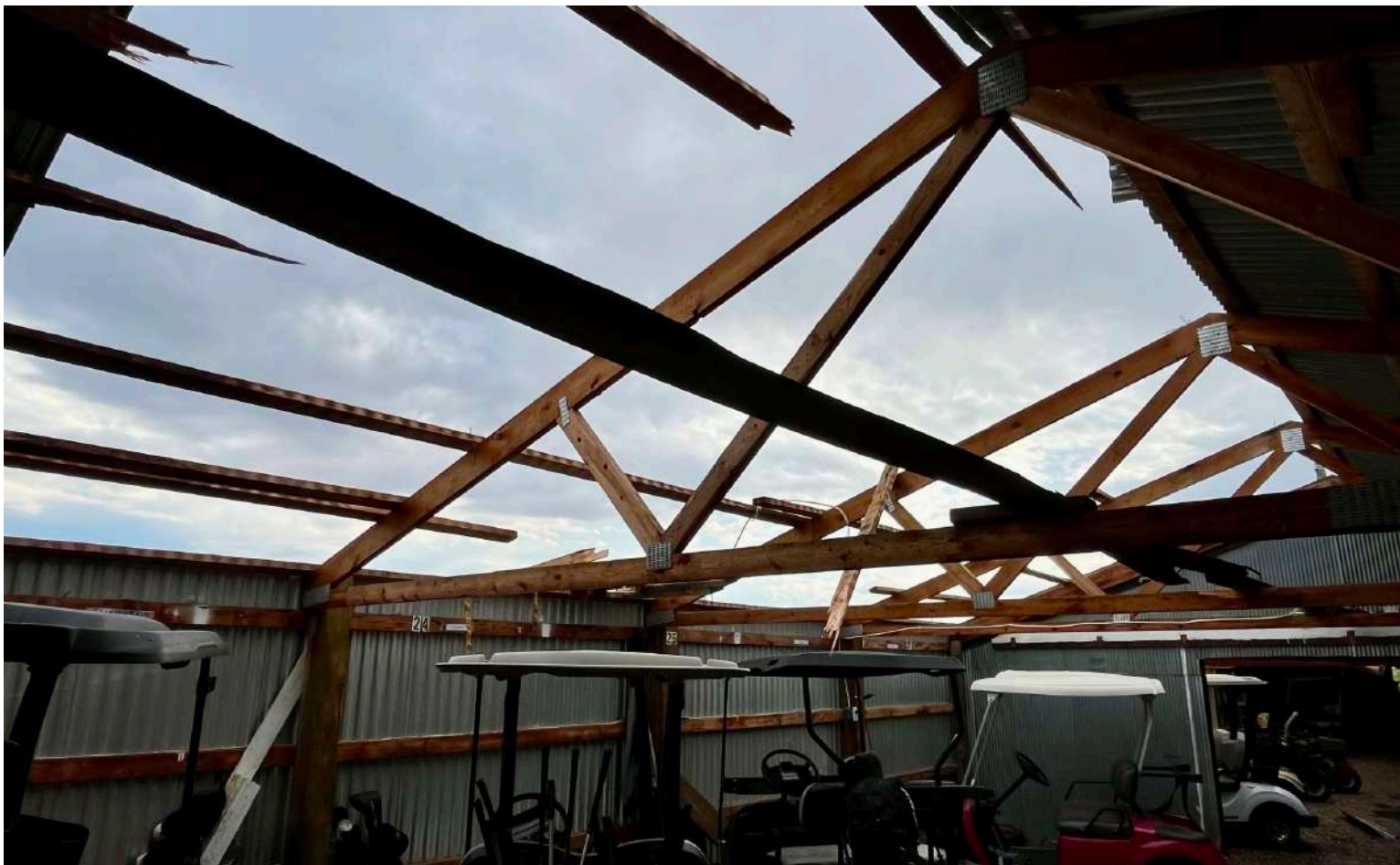
The aftermath of the storm at the Newell Golf Course. Longbrake photos
