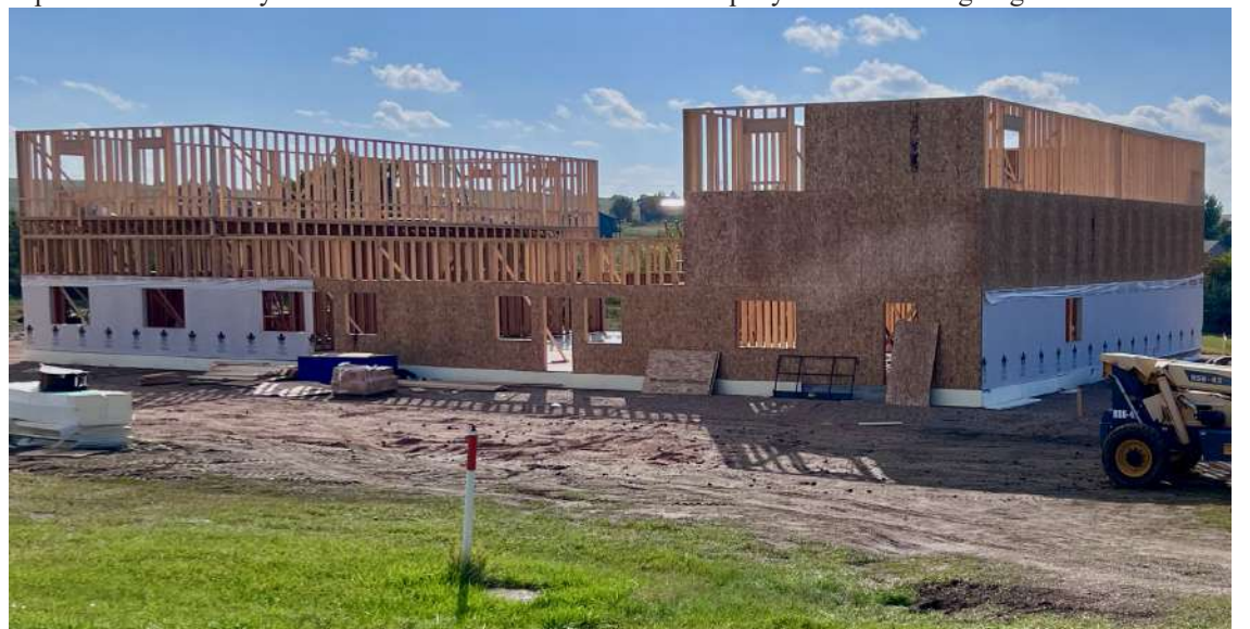
The new building going up along Highway 85 the project is being constructed by SL Builders . Longbrake photo
