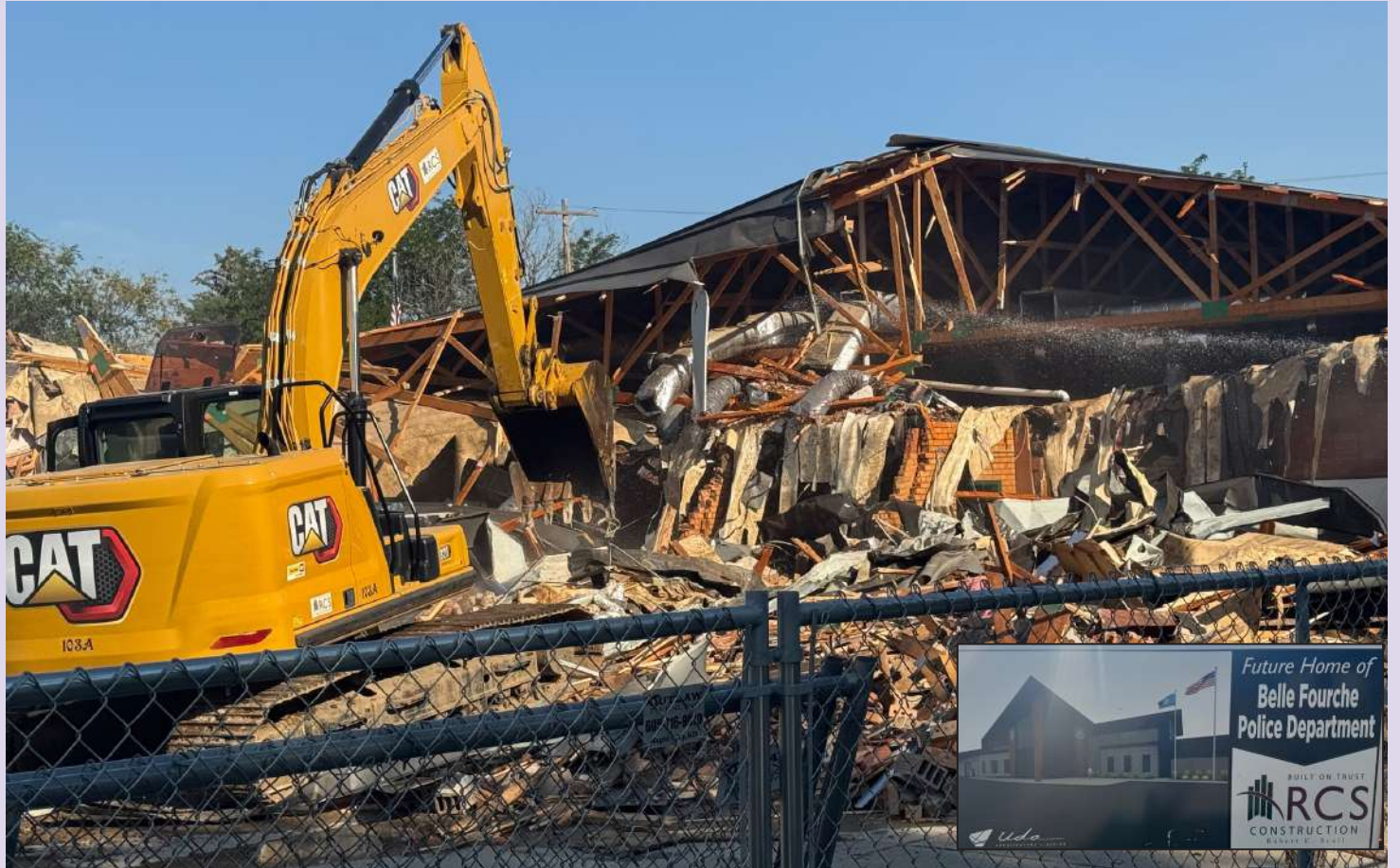
RCS Construction made short work of demolishing years of Belle Fourche History as they razed the current Police Station on the corner of 8th & Jackson (formerly elementary school-fondly referred to by past attendees as "the chicken coup". Beacon Photos
