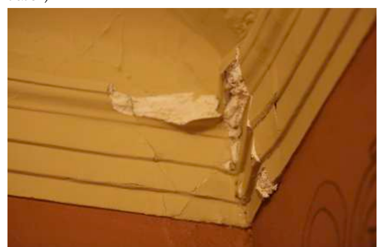
Cracked plaster in the back corner of the state House of Representatives chamber at the South Dakota Capitol in Pierre, as seen in March 2025. (Joshua Haiar/South Dakota Searchlight)
