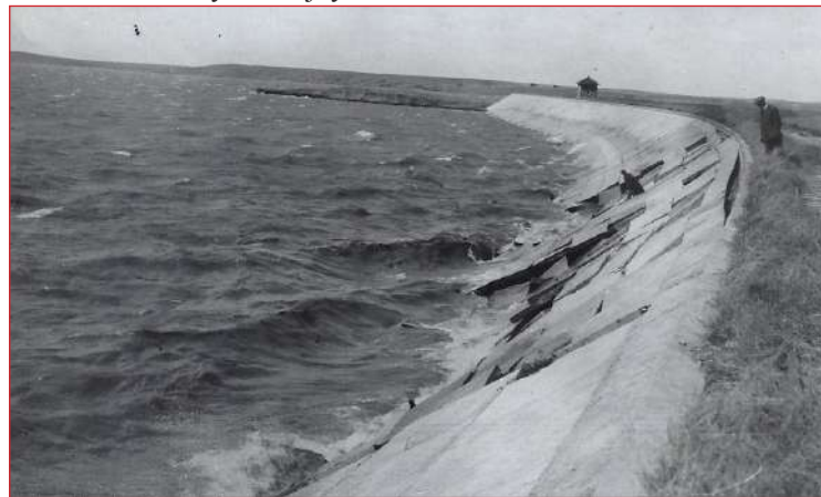
The high wave action on the face of Orman Dam pulled the concrete blocks into the dam. Newell Museum
