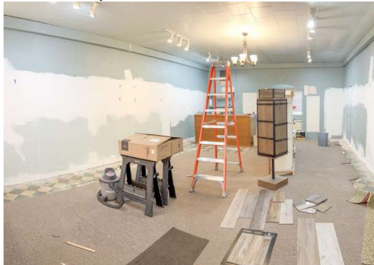
Interior renovation underway at Lifestyles soon to be Pasque Ladies Fashions. Beacon Photo
