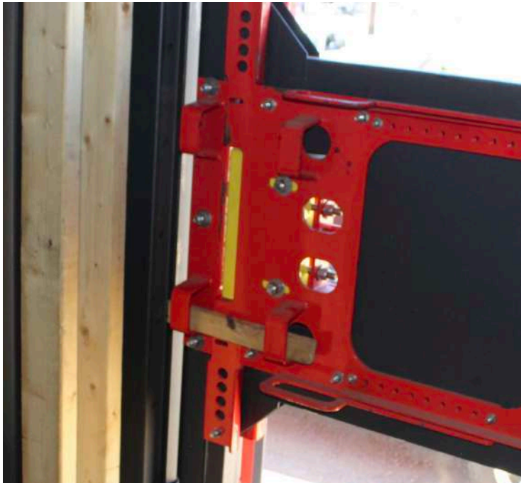
The door has a place to lock it with wooden pieces and allow the firefighters to practice breaking down the door for entry.
