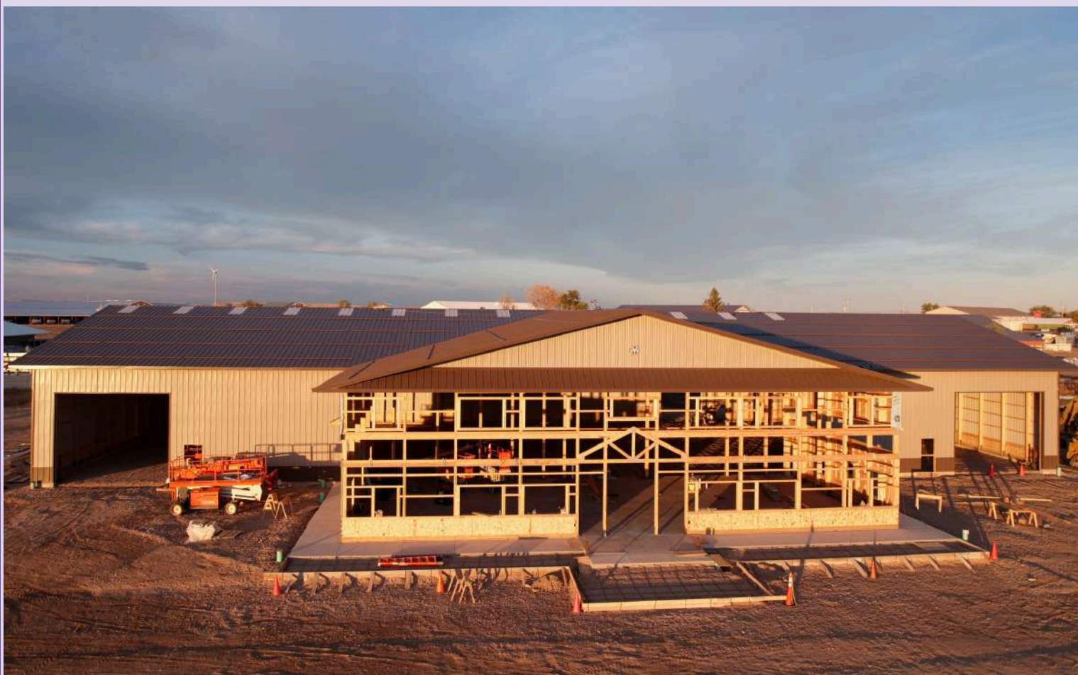
Aerial (Drone Photo) view of the CBH CO-OP facility being constructed just west of the US 85/US 212 Junction. Building will provide expanded space for Ag products, undated retail storefront and improved facilities for fuel, lube, propane, and administrative services. Hunter Anderson Photo
