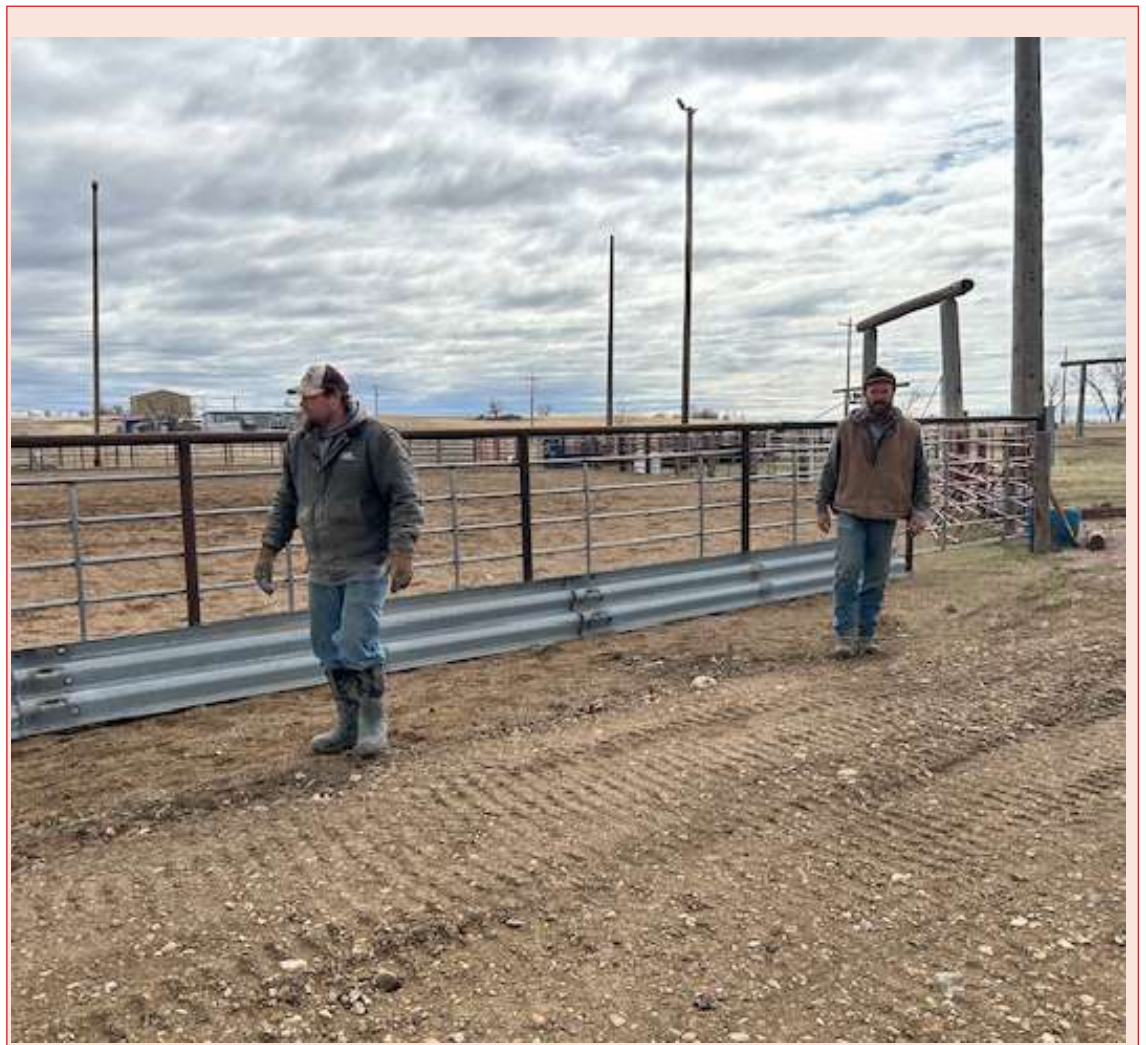
Robert Boylan and Custis Harmon welded guard rail along the bottom of the new fence at the Newell Rodeo Grounds. Courtesy Photo
