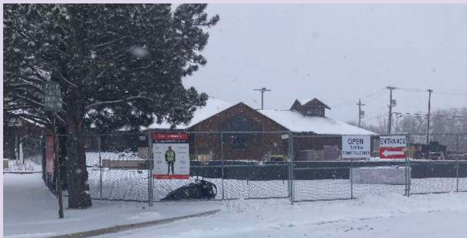
Last week's reminder of winter (the snow) brought the Tri-State Museum addition project to a halt. During more accommodating weather prior, the foundation for the addition was poured and is ready for a structure to start going up. Beacon Photo
