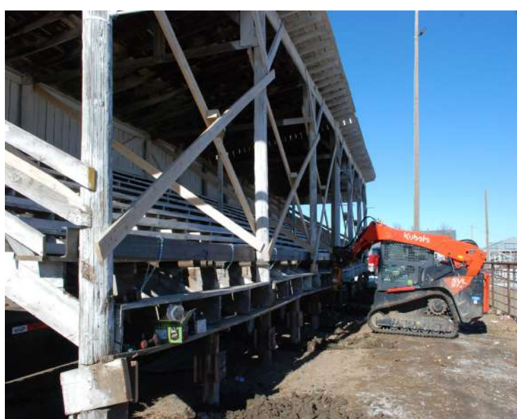
The old grandstands are gone from the Newell rodeo grounds and the new bleachers should arrive during the summer.
